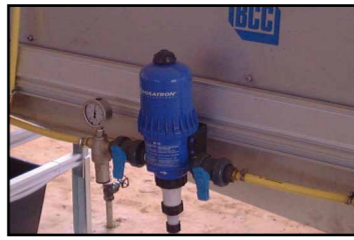
chemical dosage unit
